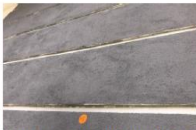
P62- Uneven paint surface on the wall
