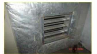
Air Handling Unit (AHU)
