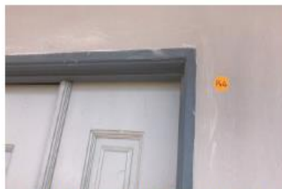
P64- Uneven paint surface on the wall
