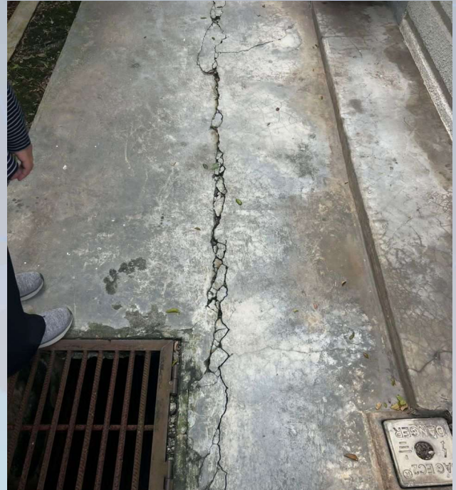
Sample of cracks on the building apron at Kolej Kristal, UiTM CPP.
